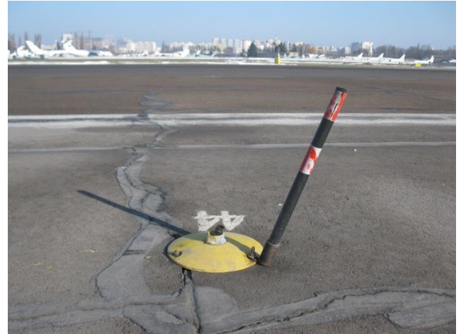
Fig. 6. Photo of the base of the attachment of destroyed runway edge light No. 44
