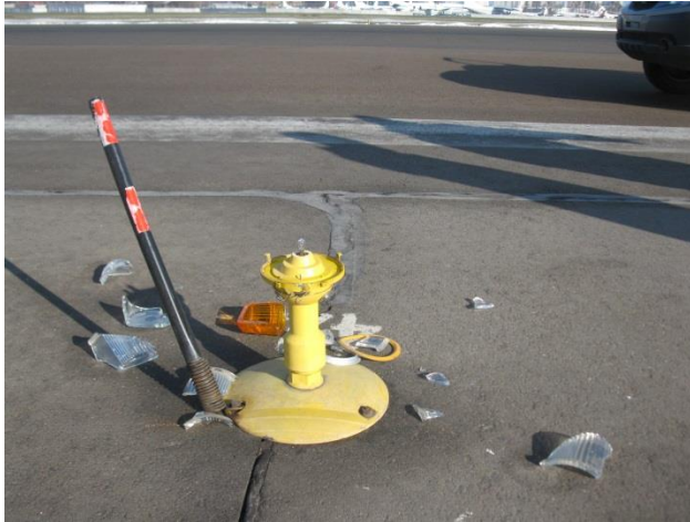
Fig. 5. Photo of damaged runway edge light No. 42
